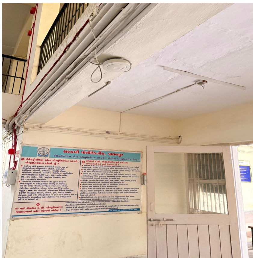
Figure 2.2.19: Departmental Wi-Fi Facility
